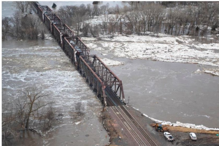
Figure 2-9: Flooded Railway Bridge
