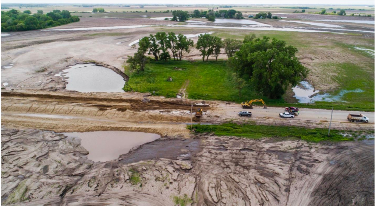
Figure 2-12: Washed-Out Road Under Repair
