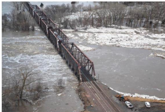
Figure 2-9: Flooded Railway Bridge
