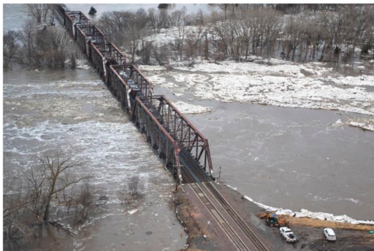
Figure 2-9: Flooded Railway Bridge
